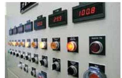
Local Operating Panel
