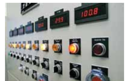
Local Operating Panel
