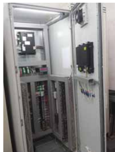
New Turbine Control Panel
