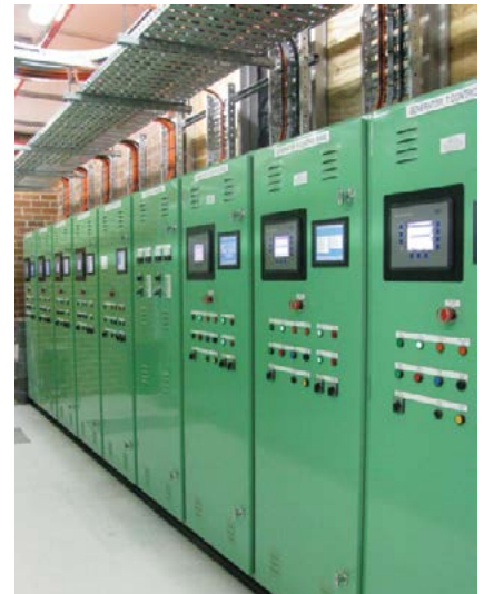
SEMS Engine control panels
